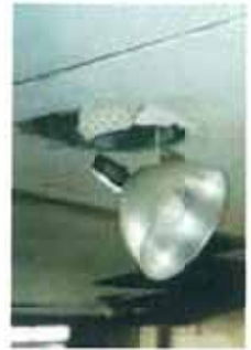
(c)照明機器の脱落
